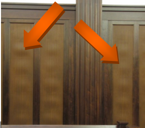
Permanent expansion to millwork panels because of HVAC system shutting down
