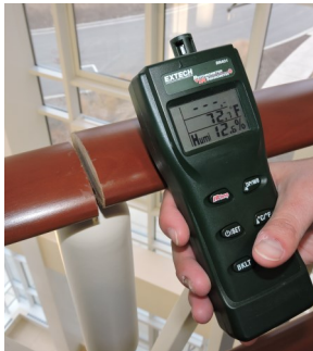
Very low humidity in the winter months created a permanent, very large gap in the railing.
